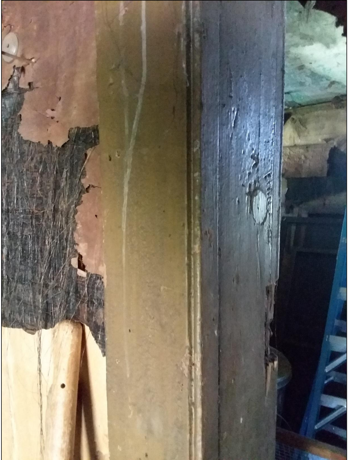
FIGURE 14: DETAIL OF TRIM AROUND INTERIOR DOORWAY, THE SAME MOLDING PATTERN AS IN THE 1856 SURGEON'S QUARTERS.
