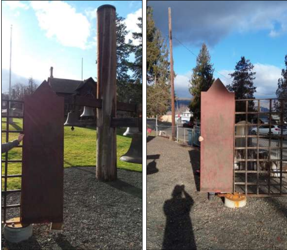
Figure 15: Mock up of the mounting boards for the interpretive signage on the Guardhouse bars.
