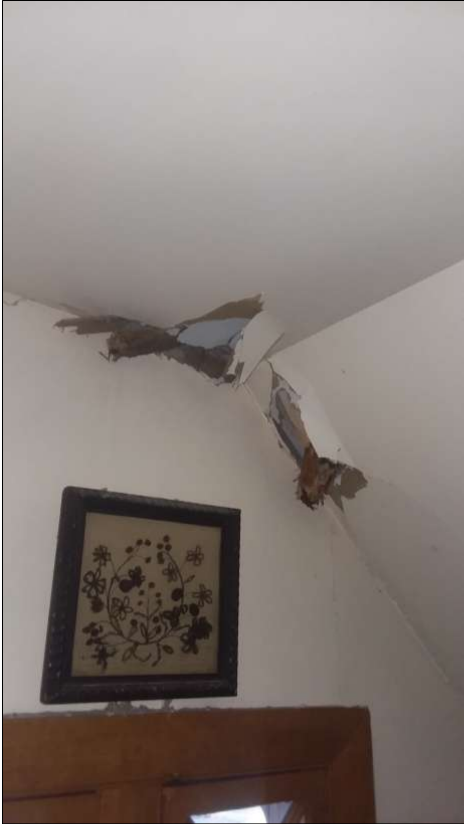
Figure 1: Branches poking through the south bedroom ceiling.
