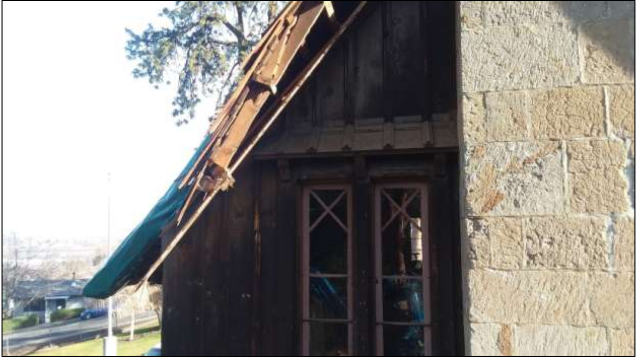
Figure 4: View from the lift of the damaged eave.
